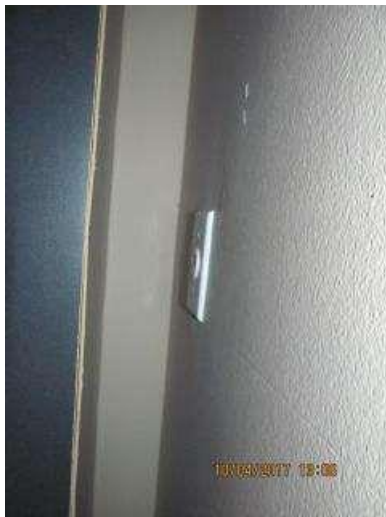
LAUNDRY ELECTRICAL - OUTLETS: The 120 volt outlet receptacle at the laundry area was not accessible and therefore not tested. Troubleshoot and repair as needed.
