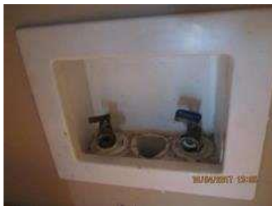
LAUNDRY PLUMBING: Water was available. Supply valves were neither moved nor tested.
